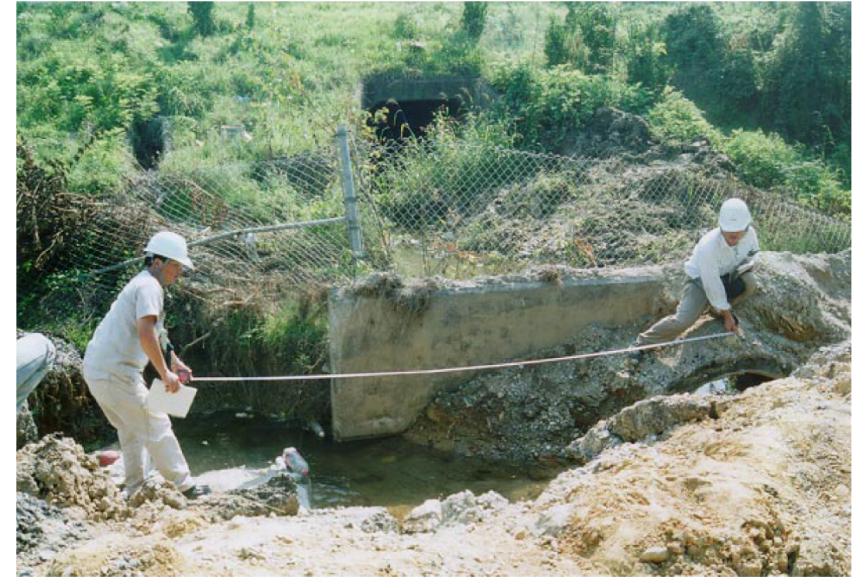
3.6 m offset of drainage Pipe (1999 Kocaeli)
